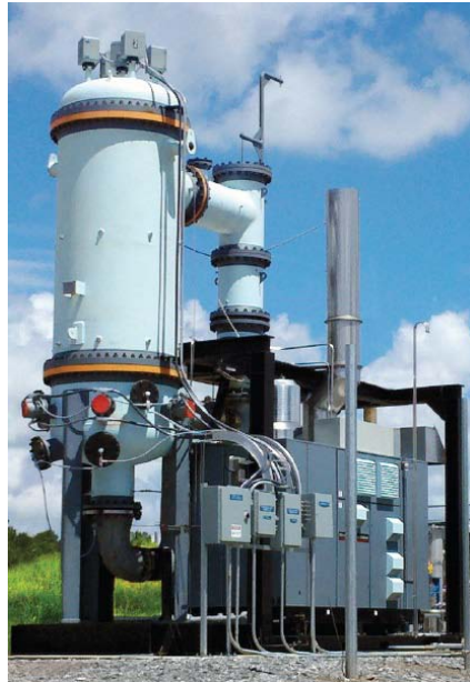
Image I. Ener-Core Powerstation FP250 Source: www.Ener-Core.com
